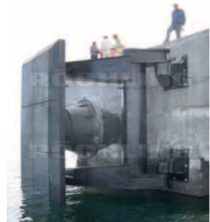
Fender on a quay wall
