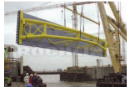
Watergate with slide rail
