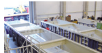
Polystone® P Random-Copolymer grey Tank for a steel-pickling plant
