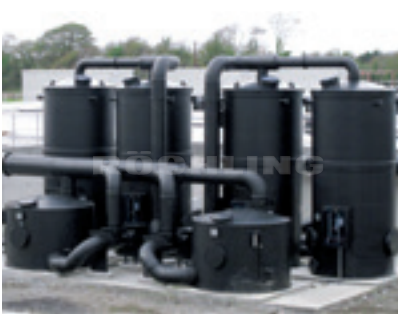
Polystone® G black B 100 Air purification system in a water treatment plant
