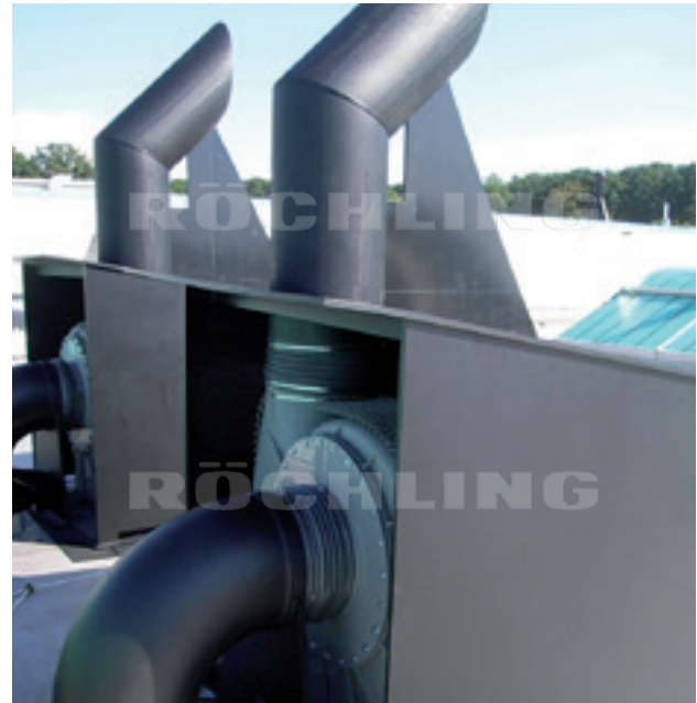
Polystone® G HD black Housing of a ventilation plant on a hall roof. Here, good weather resistance is absolutely essential.
