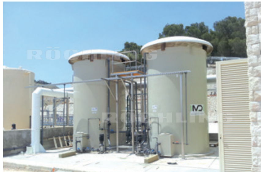
Bio filters for odor neutralisation
