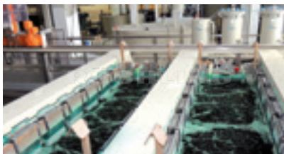
Tanks made from Polystone® P in a plastic electroplating plant
