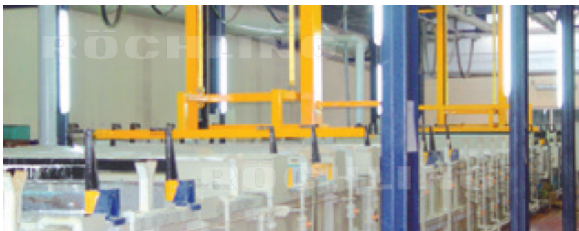
Polystone® P homopolymer grey Galvanic plant for the treatment of aluminium parts
