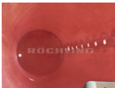
Trovidur® NL Inliner in a distillation column (interior view)
